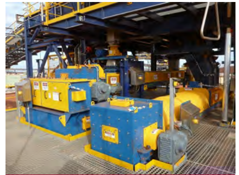
Consep's sample crushing, feeder and integrated linear sampler arrangement
