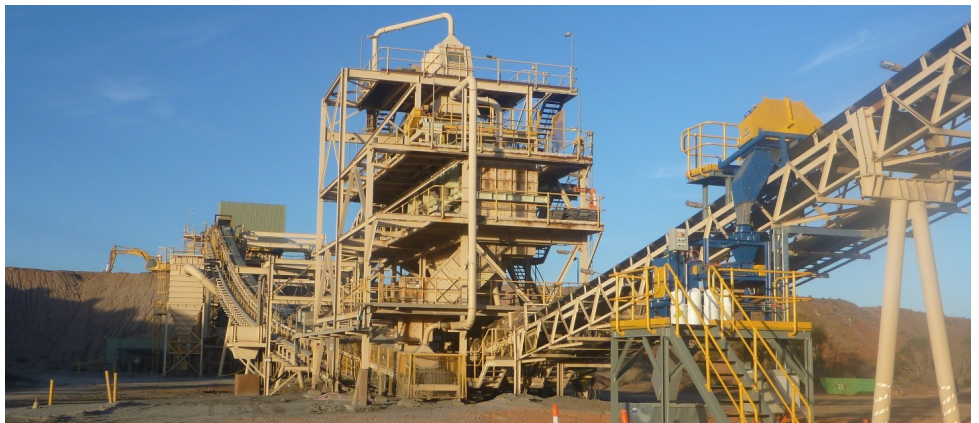
Carosue Dam's Crushed Ore Sampling Station
